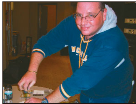
Tocco puts the cover back on the Omnia-6 after the firmware card replacement.
